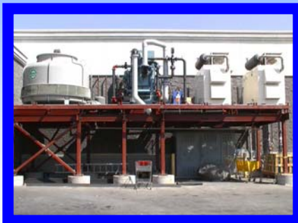
Combined Heat and Power
